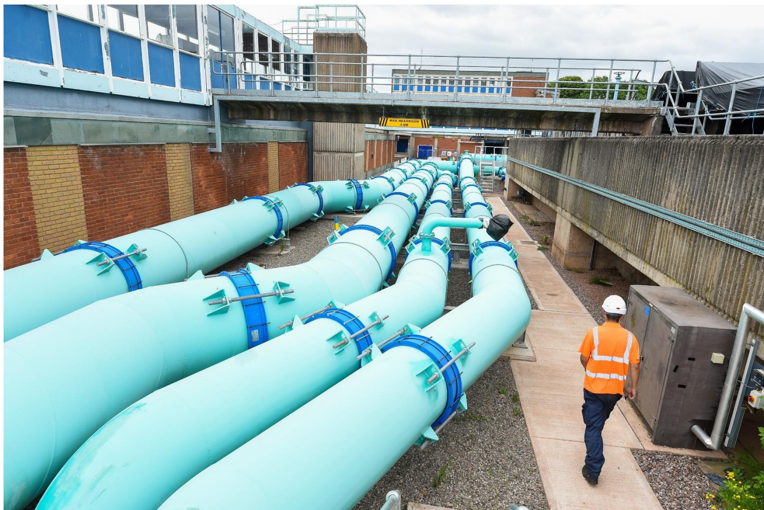
New pipe configuration at the Hampton Loade water treatment works, July 2022. Photo: Carl Murphy
